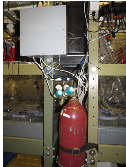
Carbon Dioxide Tank
